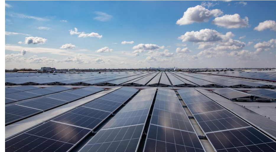
Solar panel field
